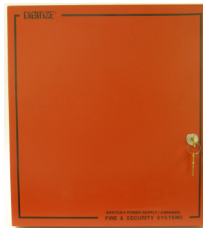
KRATOS-4 Power supply charger and battery box
