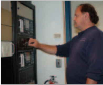
Terry Freund, program manager for Fire Protection and Emergency Services at Cornell, says the upgraded alarm system provides critical information such as the exact location of the alarm within the building and conditions that responders might expect to find.
